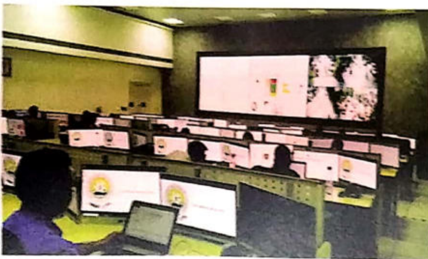
City Operation Center, Visakhapatnam Smart City
