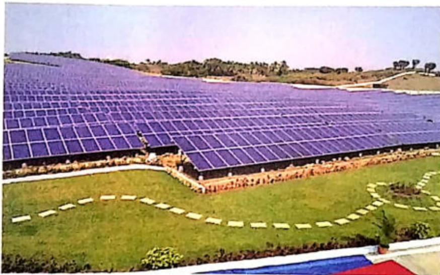
Solar PV Installation, Diu Smart City
